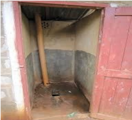
Ventilated Improved Pit (VIP) latrine 2
