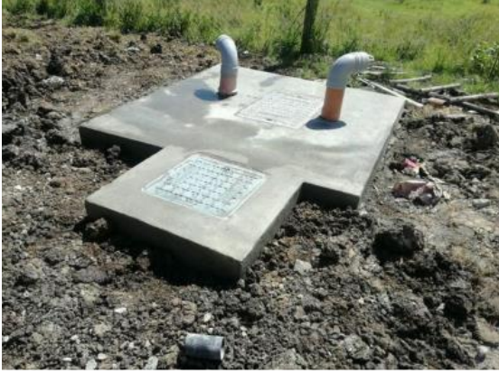
Biodigester Septic Tank
